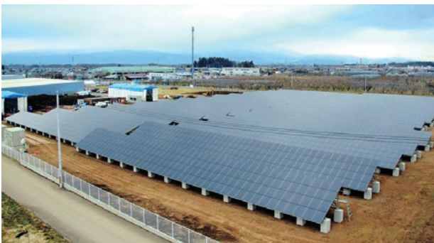
System installed at Yamagata Factory in 2013 (capacity: 732 kWh)
